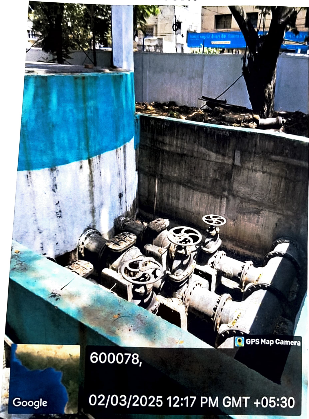
K.K.Nagar "A" SPS Newly constructed at Alagirisamy salai
